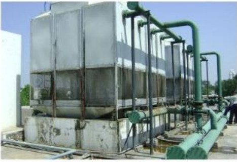
The Delhi Metro Station Cooling Towers
