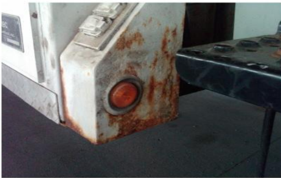
Power Dist Box - Before Rust Bullet Application
