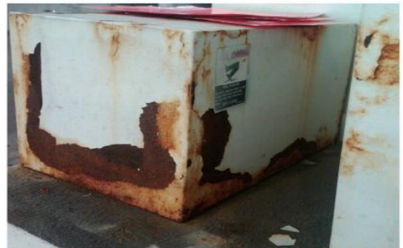
Radar Box - Before Rust Bullet Application
