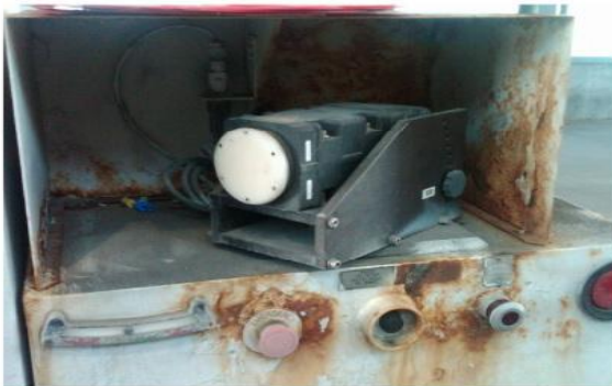
Radar Box - Before Rust Bullet Application
