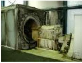
Gas Turbine Air Inlet Plenum
